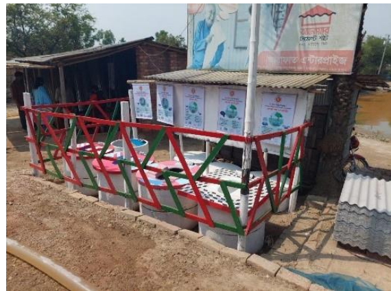
Figure 3: Demonstration of stacked pre-cast concrete rings to elevate latrine pit by latrine producers, Bangladesh, 2020
