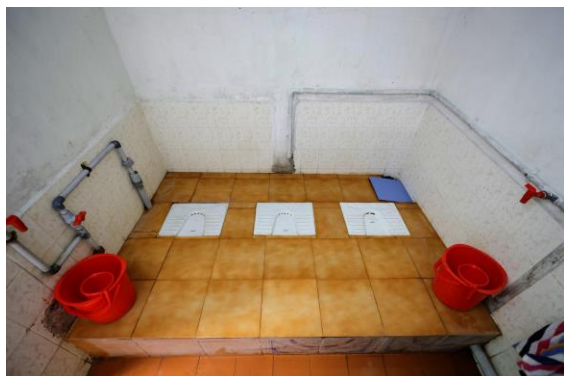
Figure 5: Water storage for toilet flushing
