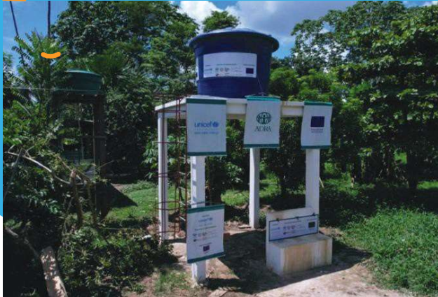
Alternative Collective Solution of Water Supply for human consumption (SAC) implemented in indigenous community in the DSEI/ARS – December 2022.
