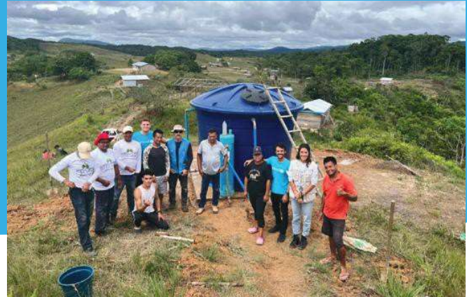
Treatment and distribution system for safe drinking water in the Sakao-Mota community of the São Marcos indigenous land, in partnership with CIR and DSEI-L/RR, Pacaraima/RR – January 2023.
