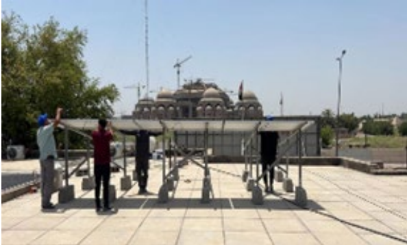
Figure 5: Installation of solar panel in Al Hijrah school-Baghdad, 2023 photo captured by UNICEF consultant
