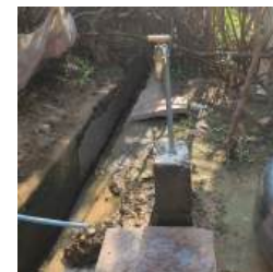
Presence of FHTC within 2 meter of drainage in Gadwas Village
