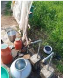
FHTCs are placed outside the house (Gadwas Village)
