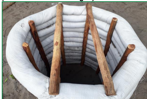
Figure 1: Low-cost lining – suited to wet, unstable sand found in Western Province (one of 5 different designs)
