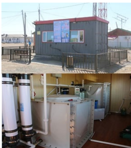
Figure 7: Smart water kiosk in Khukhmorit sub-province and water purification filters installed inside the kiosk.
