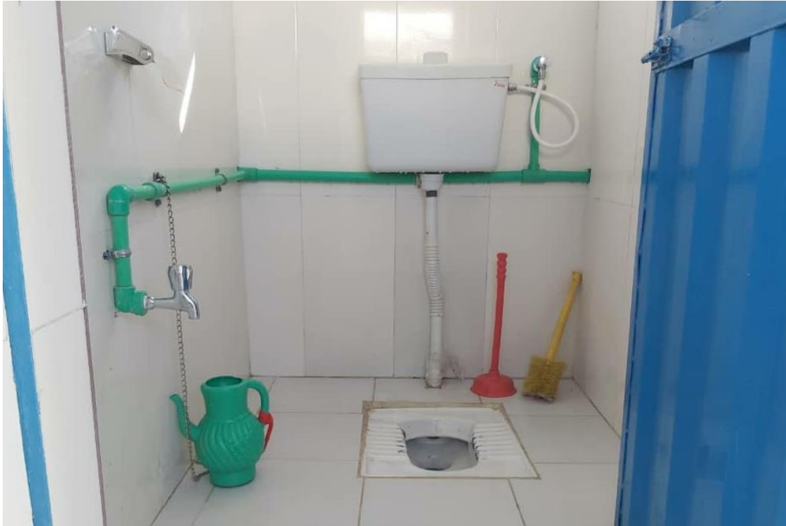
Picture 3: Constructed eco-friendly flush latrines for the school students (Source: Afghanistan WASH team).
