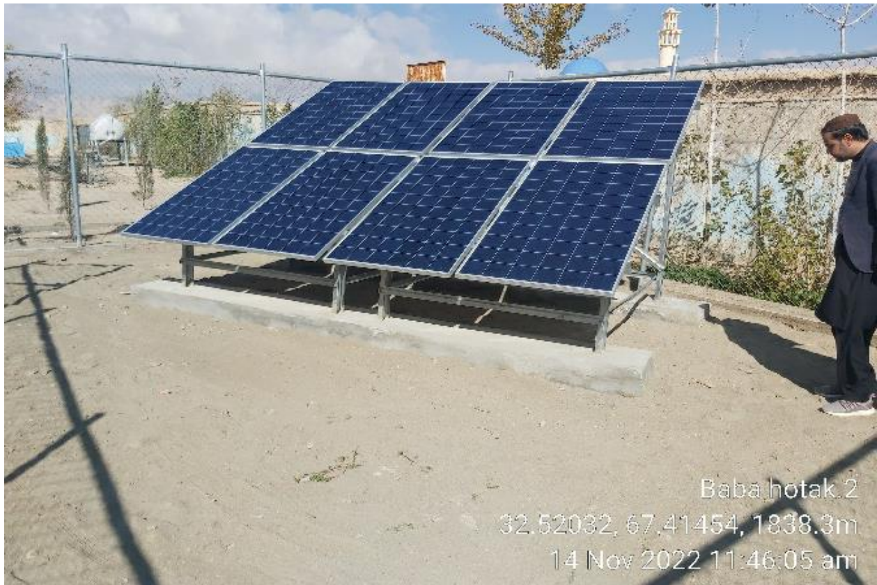
Picture 2: Installation of solar powered water supply system (Source: Afghanistan WASH team).
