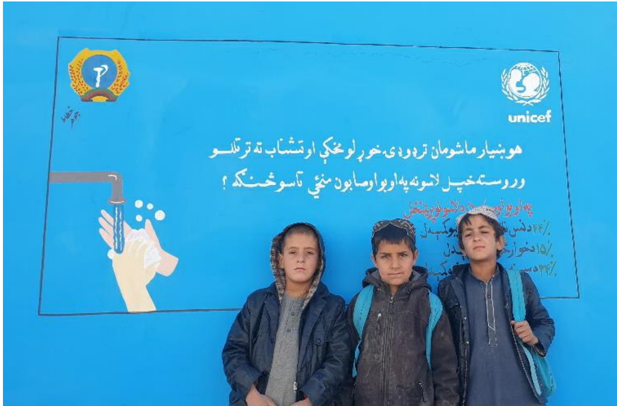
School students expressing their joy standing next to newly constructed toilets. (Source: Afghanistan WASH team)
