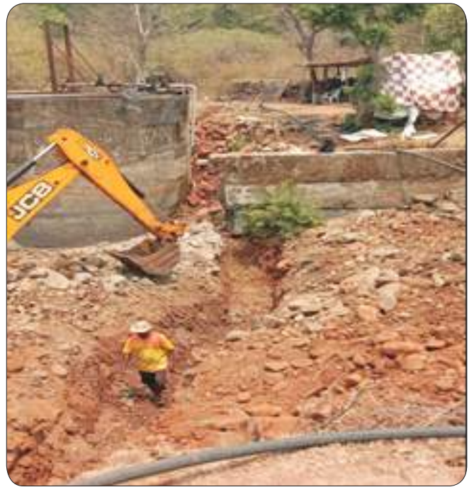
Pipelines laid under river bed after floods in Talsar Village, Chiplun Taluka, Ratnagiri District
