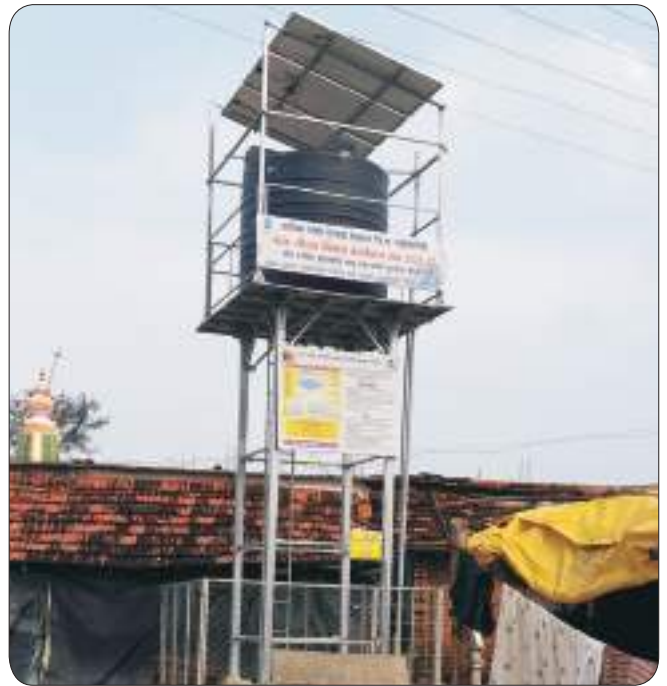
Solar-based drinking water scheme installed under the Jal Jeevan Mission at Usegaon Village, Gadchiroli Taluka, Gadchiroli District
