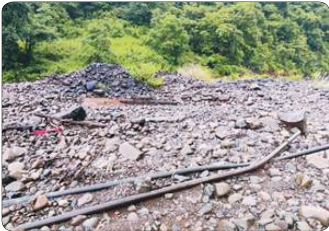
Well damaged due to floods in Posare Village, Khed Taluka, Ratnagiri District
