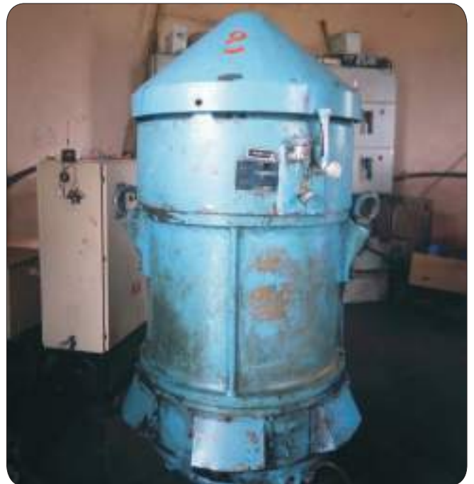
75 HP pump damaged in the flood
