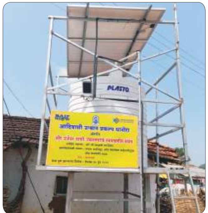
Solar-based drinking water scheme installed in Pandarsara Village, Kurkheda Taluka, Gadchiroli District
