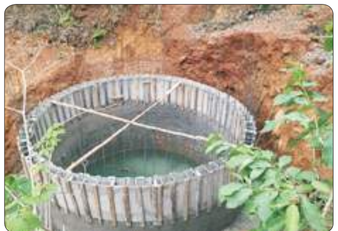
Construction of new well with modifications in Vetoshi Village, Ratnagiri Taluka, Ratnagiri District
