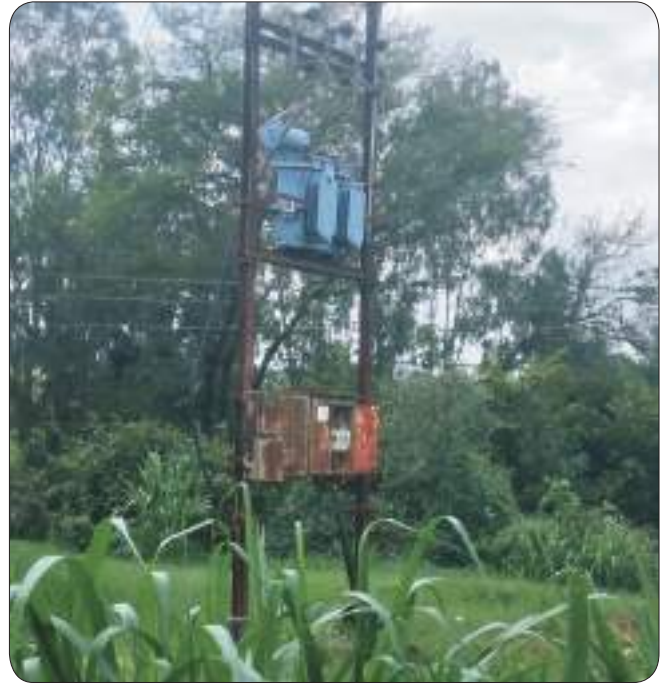
Villagers faced electricity supply issues in Kolhapur
