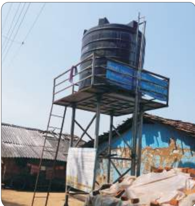
Solar-based drinking water scheme installed by GDSA and an NGO in Gadchiroli District
