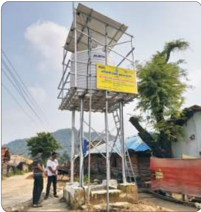
Solar-based drinking water scheme installed under the Jal Jeevan Mission at Kakadayeli Village, Dhanora Taluka, Gadchiroli District
