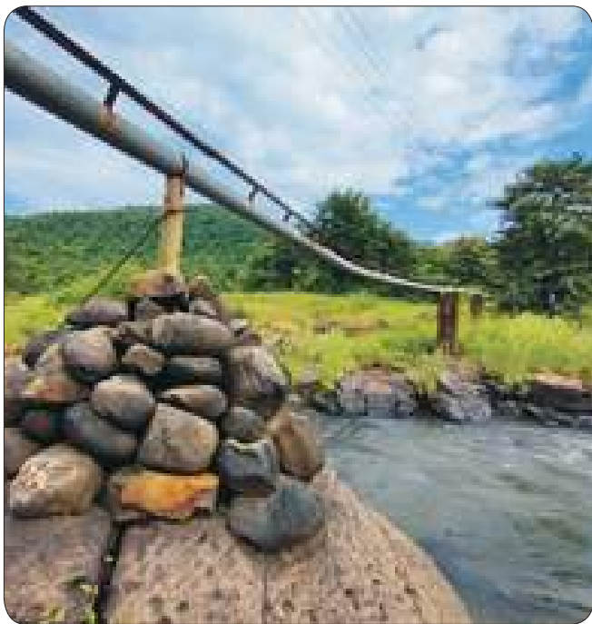
Pipeline height raised above the flood level in Talsar Village, Chiplun Taluka, Ratnagiri District
