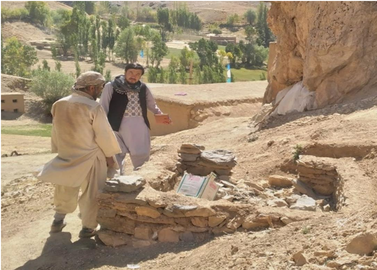
Construction of latrine after attending the sessions by the CLTS team in Joqul village in Waras district
