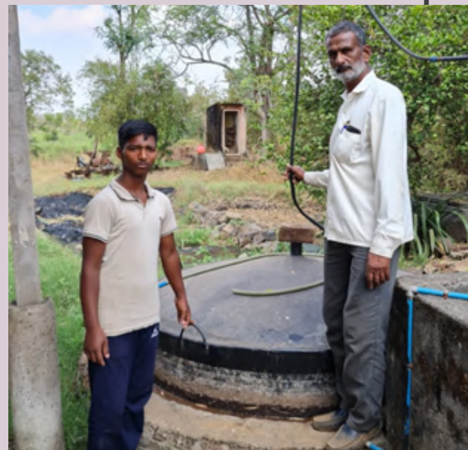
INDIVIDUAL LEVEL BIOGAS PLANT
