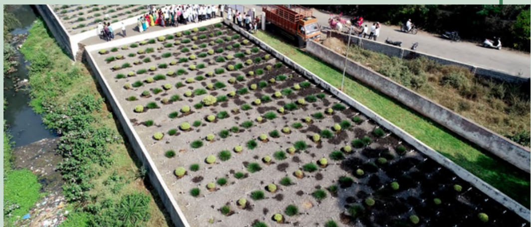
STP AT KUNDAL GP
