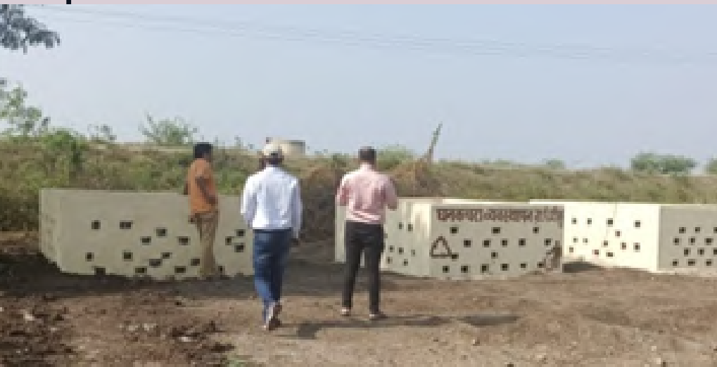
WASTE COMPOSTING UNIT
