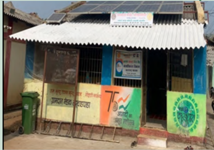
INSTALLED SOLAR PANELS
