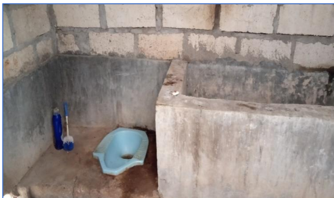
Picture 1 Toilet at a Rural Puskesmas, Southwest Sumba East Nusa Tenggara
